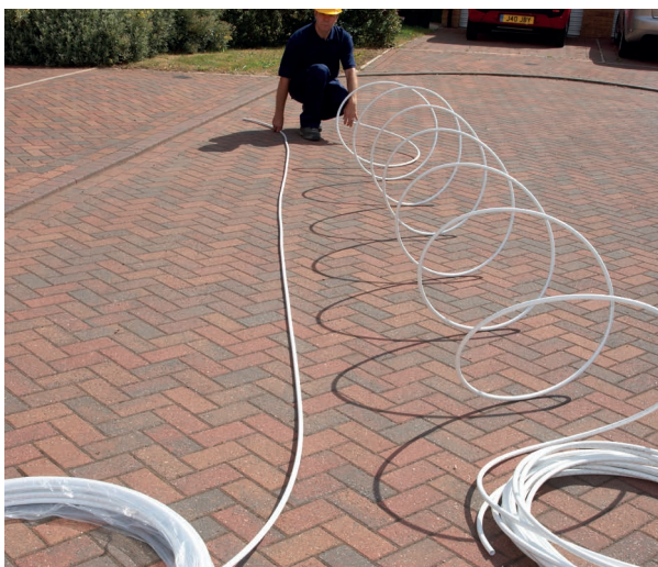
Fig. 4 Hep 2 O pipe (left) comes off the coil straight
