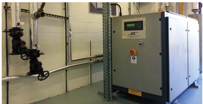
CHP plant room, Telford
