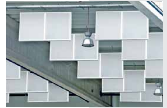
Optimised plant acoustics thanks to TROX splitters
