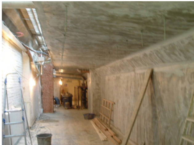
Triton Fillet Seal used to form wall to soffit junction in basement renovation
