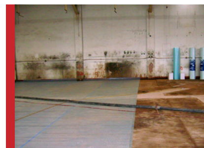
Platon Multi used as barrier against contaminated substrate in renovation of industrial building
