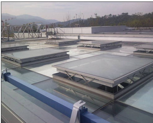
An example of Parallel Plus used on rooftops.
