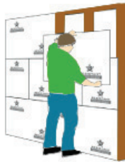
4. Offset boards when fixing. Four corners should never meet. The tiling side (coarse side) is marked on all boards.
