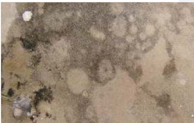
▲ Mould/fungi on plaster board
