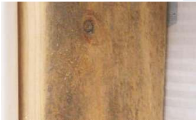
▲ Mould/fungi on timber stud in the cavity
