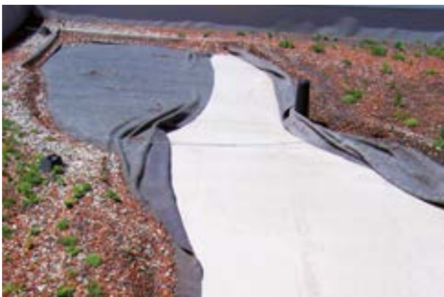
▲ Wind erosion, in this case all the way down to the roof waterproofing
