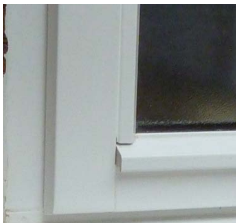
Modern storm-proof casement detail with incorrect rebated openers lipping over the face of the frame
