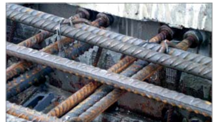
Exact reinforcement layer in the 2nd concreting phase due to simple installation of the Coupler connecting rods in the indented joint.
