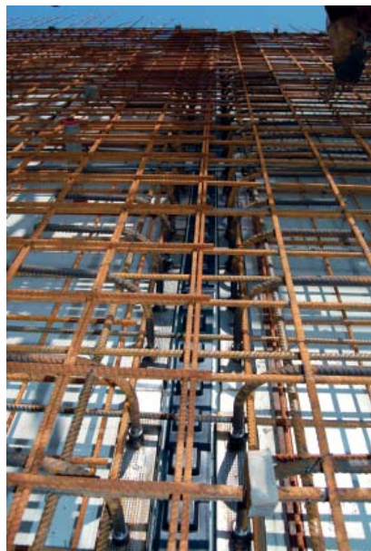
Reinforcement layer in the 1st CP: attachment of the WCA coupling bars to the local reinforcement
