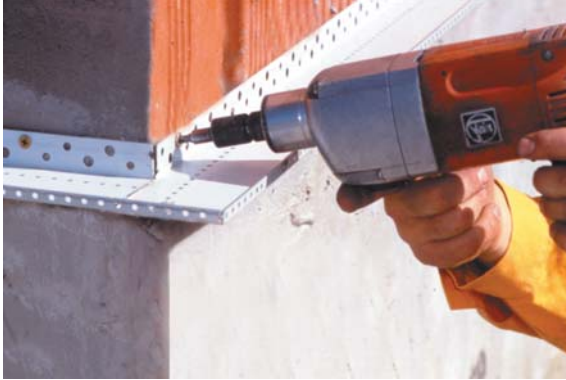
The base trough profile is used to form the base terminator. It is aligned using a string and fastened to the masonry with dowels.
