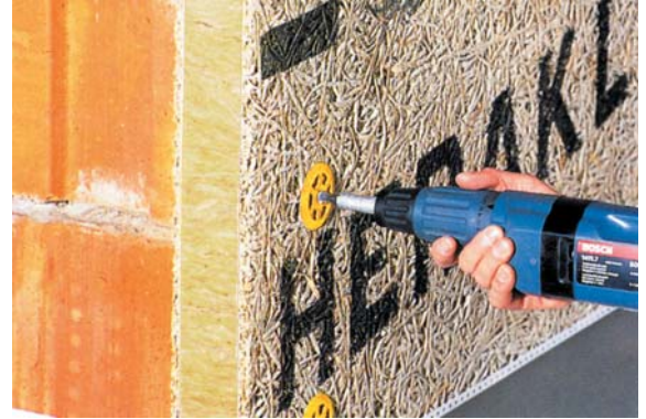
The first Tektalan-E-21 board is placed on the base trough profile and fastened with a Heraklith "E" dowel in the middle of the board.
