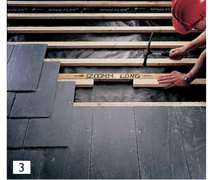
3 Fix an additional 1.2m support batten above the cut batten (spanning two rafters) and nail to the adjacent rafters.
