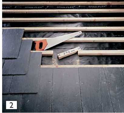
2 Use the trimmed slates to mark a 270mm long gap in the middle batten. Cut out this section of batten.
