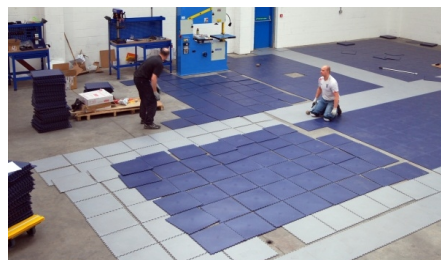
Pic 4. Split the pallet and spread the tiles across the floor prior to starting installation.
