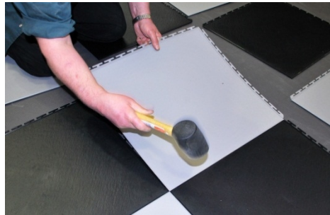
Pic 5. Don't force the tiles, offer up the corner of the tile and gently hammer the joints together.
