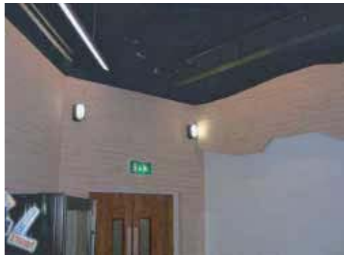
SP Maintained Emergency luminaires installed throughout an entertainment centre
