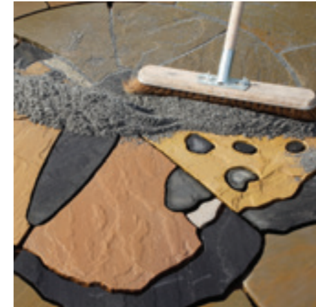
4. The material is brushed into the joints ensuring the joint voids are full, and any excess brushed off.
