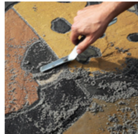
5. The joints are struck off using a pointing iron. Any gaps that are revealed are refilled with Fast Point.
