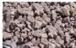
Lower Layer 250mm depth 10 - 63mm clean crushed stone with well defined edges.
