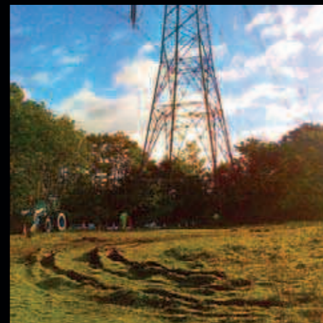
Rigging a pylon - without Ground-Guards!
