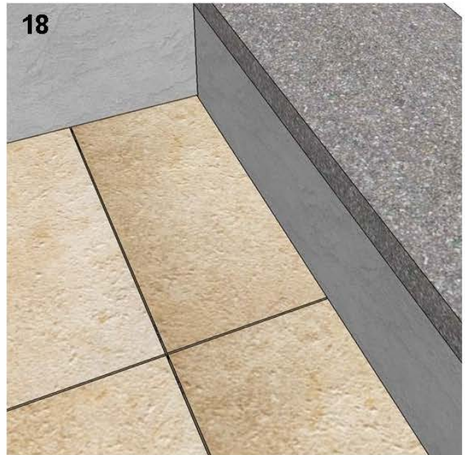
18 - Continue laying the pedestals and cut slabs in the same manner to all remaining edges requiring cut slabs.
