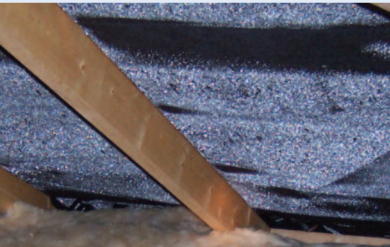
Impermeable underlay (type HR) with flocked underside showing condensate being held
