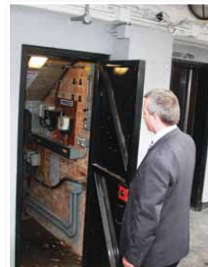
The electrical intake service rooms remain clean and functional upon inspection.
