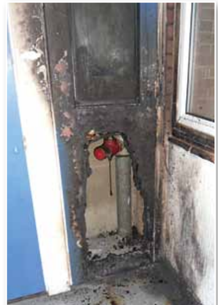
A fire door (non Gerda fire door) subject to arson, exposing the dry riser - important equipment that the Fire & Rescue Service needs in full functioning order.
