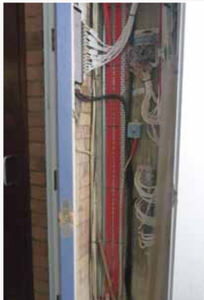
A breached fire door (non Gerda fire door) exposing the contents of the electrical intake cupboard which, if damaged, could significantly affect the building.
