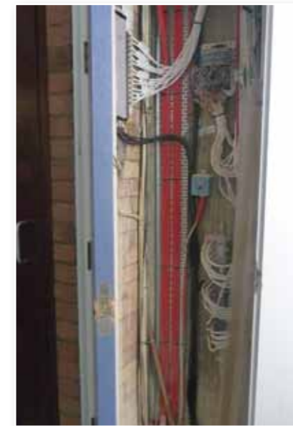
A breached fire door (non Gerda fire door) exposing the contents of the electrical intake cupboard which, if damaged, could significantly affect the building.
