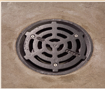
Ductile iron circular grating in a concrete floor
