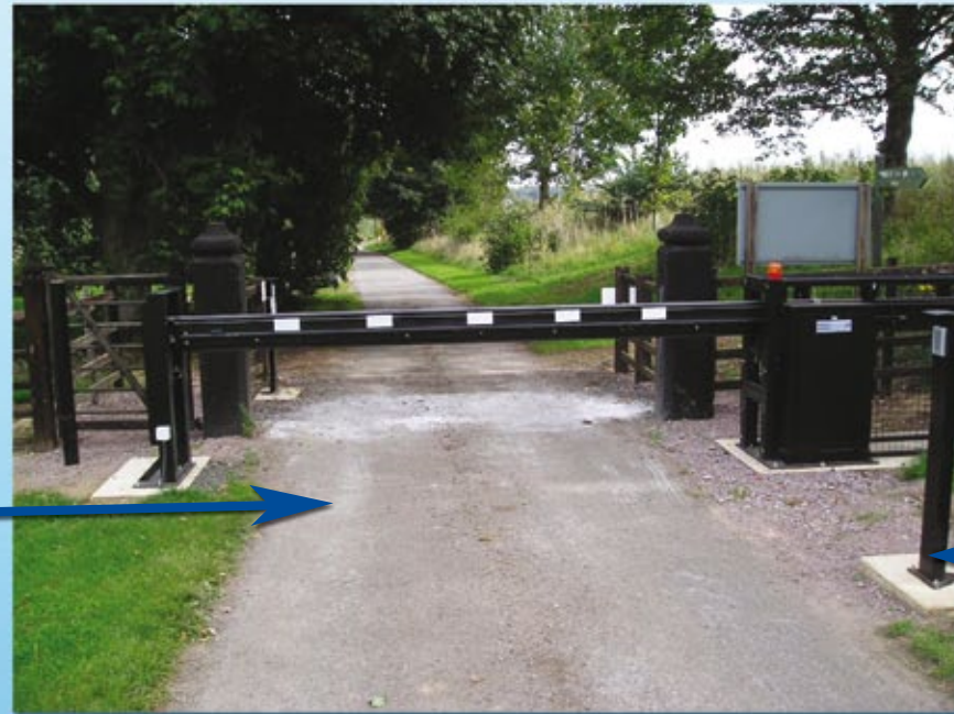
Vehicle Detector Loop laid in the road surface
