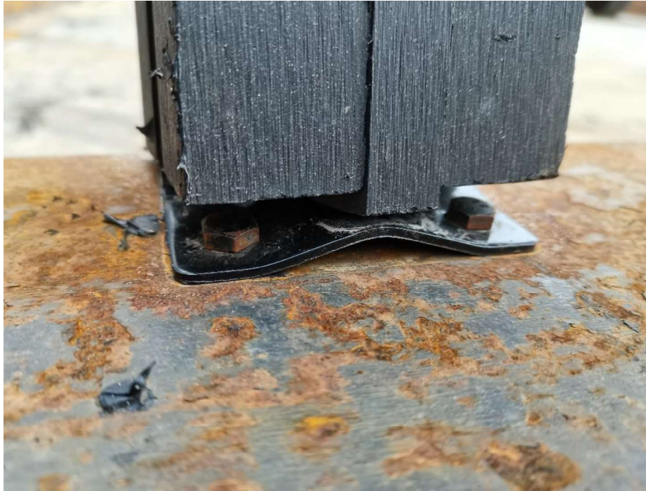
Photo No.5 The feet of fence were damaged at wind speed of 77 mph for 47 seconds
