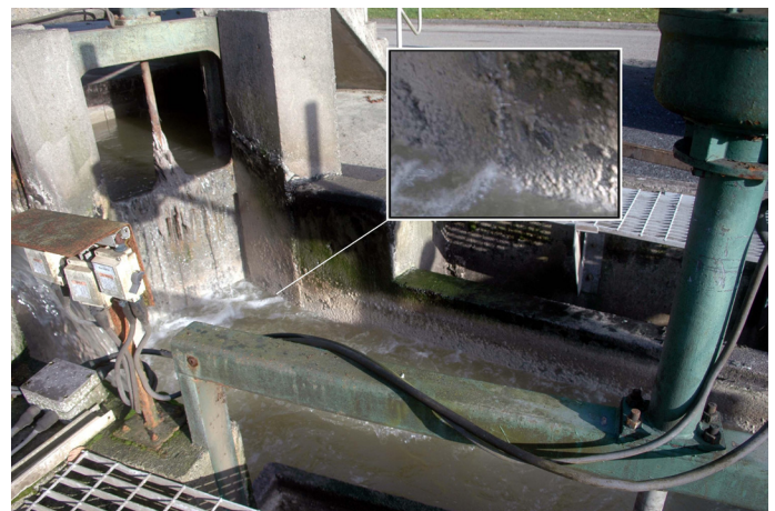
Gypsum formation above the water line
