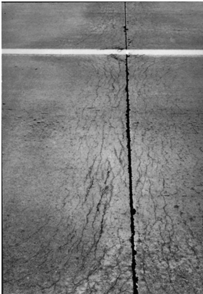
D-Cracking due to freeze-thaw attack
