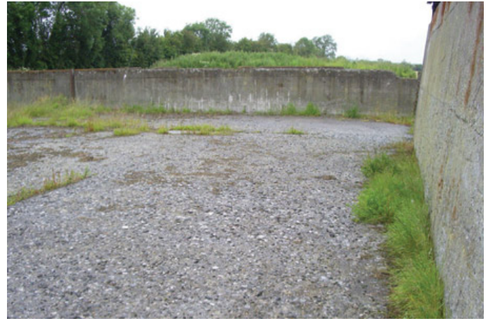
Silage pit where concrete has been damaged as a result of exposure to silage effluent acids
