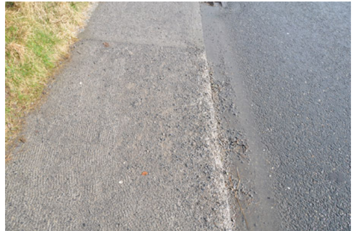
Scaling and delamination due to freeze-thaw attack (note small size of aggregate)
