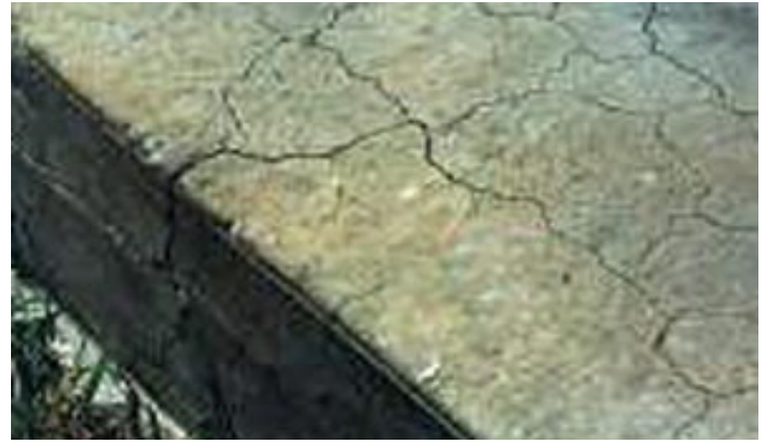
Concrete suffering ASR degradation
