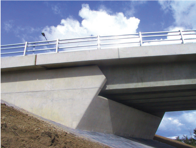
Concrete bridge abutment made with 50% Ecocem GGBS; bridge beams are made with 100% OPC.
