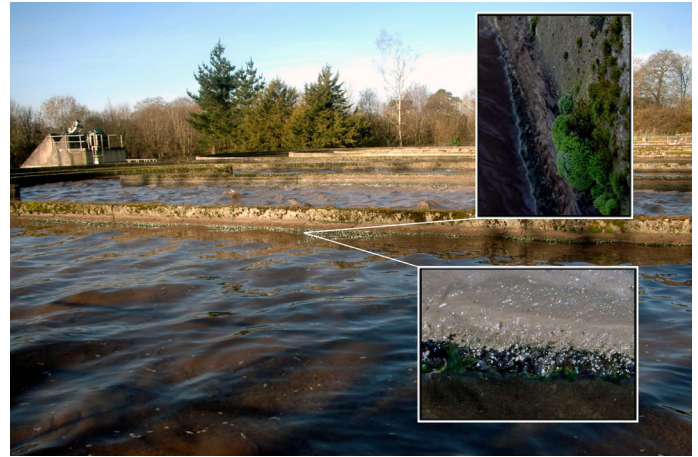
Acid erosion of cement matrix leading to exposed aggregate
