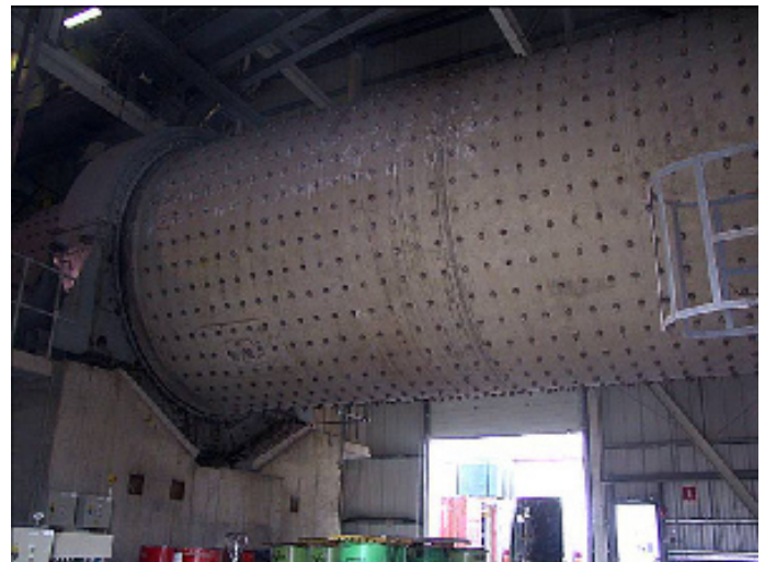
The granulated slag, after drying, is ground to a very fine powder in the rotating ball mill, which contains some 3.6 million high chromium cast steel balls.
