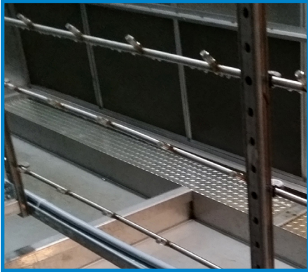
Atomizing nozzles upstream from air filters
