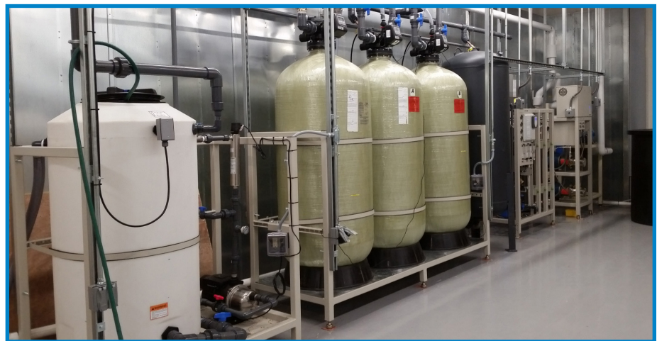
Reclaim tank (far left) for water that does not evaporate in the air handlers
