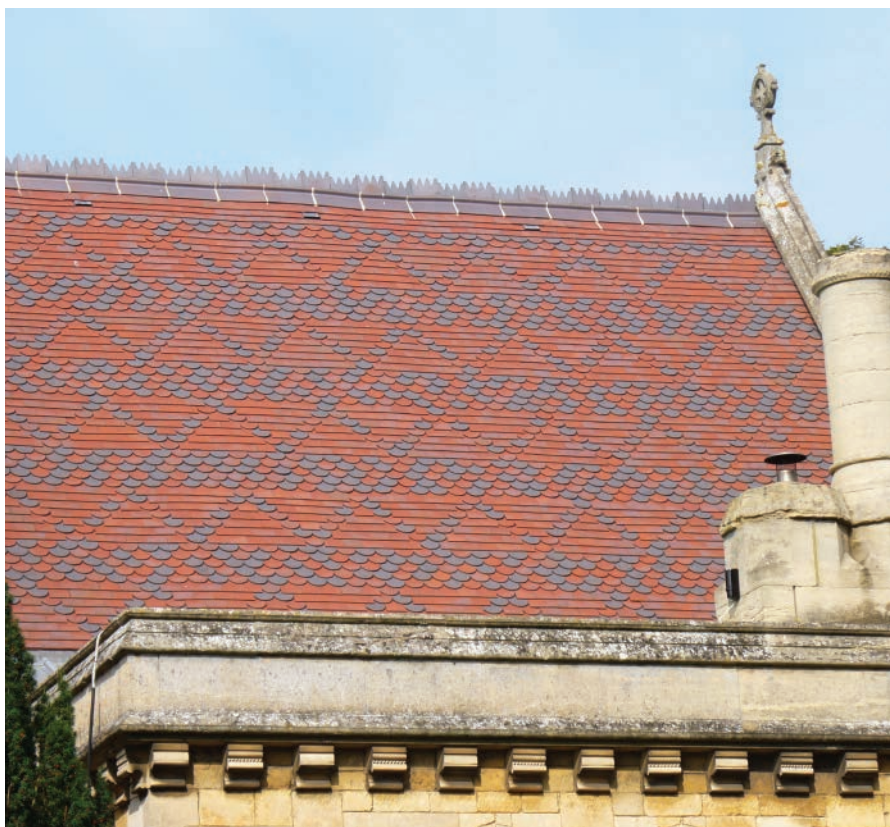
Above: Ornamental tiles in Red Blue Blend and Staffordshire Blue were used to recreate the polychromatic diaper pattern on this Gothic Revival church.
