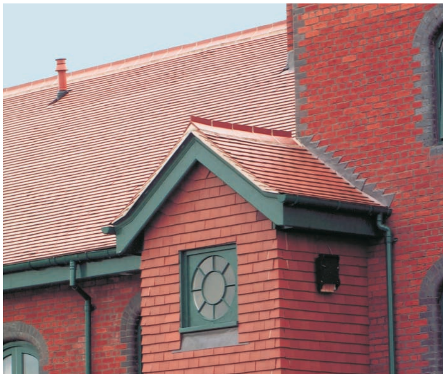
Right: Mossley Hill Hospital Liverpool Plum Red tiles were used to re-roof this Nineteenth Century Hospital, special interlocking Ridge Tiles were made to match the originals.
