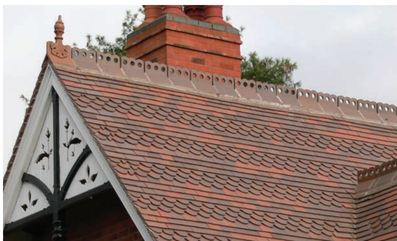
Above: This Victorian House was re-roofed using a mixture of Brown Brindle and Country Brown Tiles with Ornamental Club Tiles to match the original. Ornamental finials and ridge tiles were hand-made to match the original.
