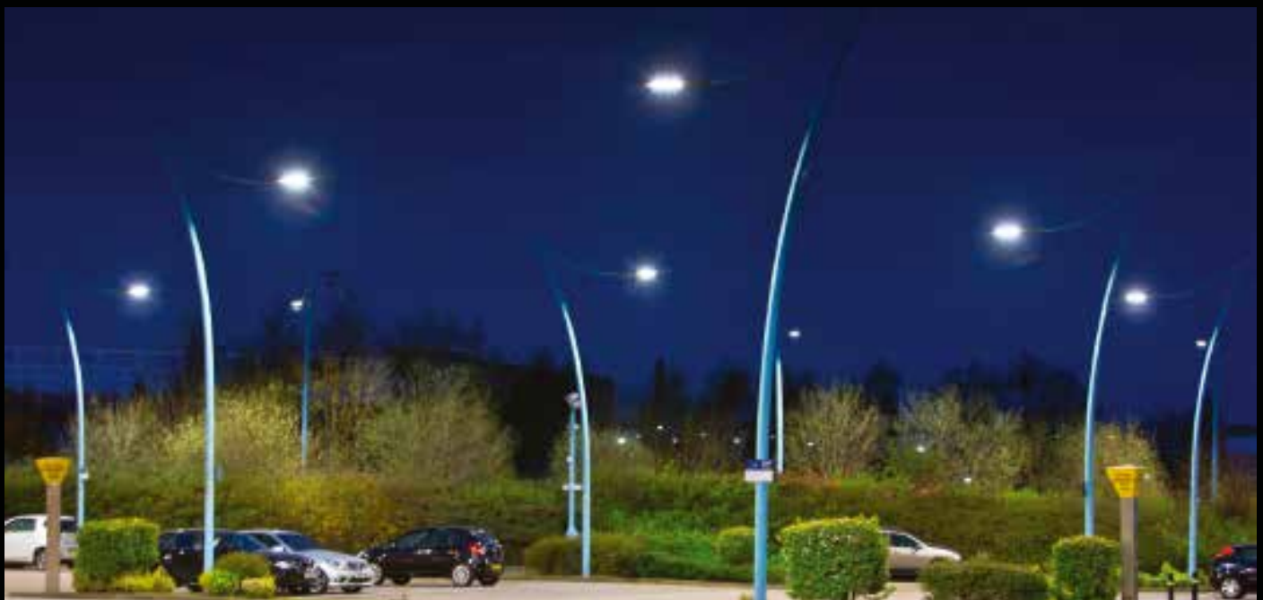
Hawthrones Car Park - CU Phosco P850 LED Lanterns installed by others
