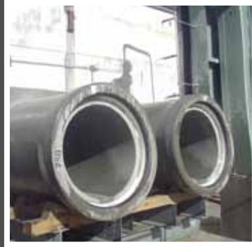
CPM has invested in the only 'rope' saw of its kind currently working in the UK, which can cut multiple pipes
