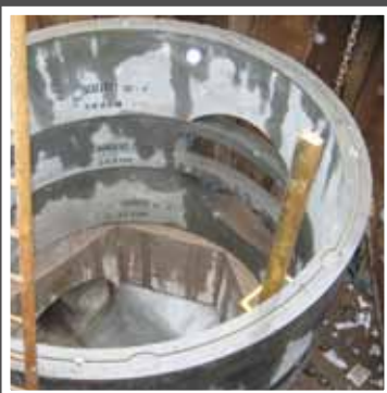
3000mm sectional chamber installation with a letter box opening for 1500mm concrete pipe.
