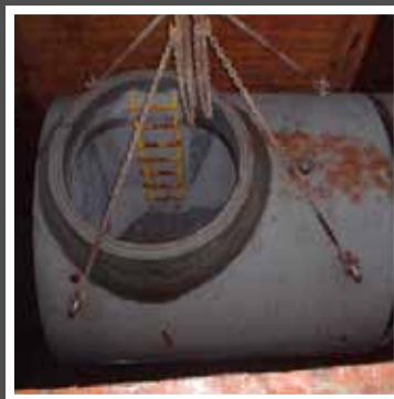
End entry pipe
