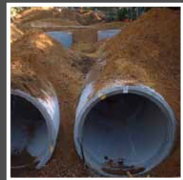
Side entry manholes
