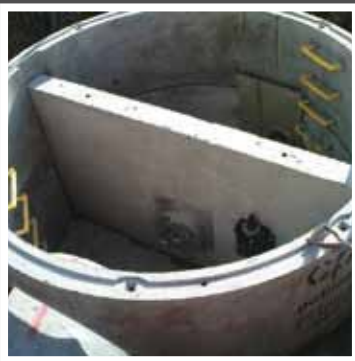
2550mm wide wall chamber installed complete with Hydro-Brake® and penstock on weir wall.
