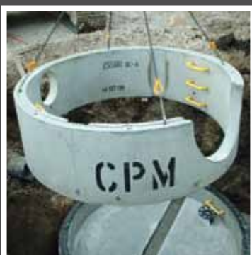
2550mm sectional installation, upper ring with half formed hole for 900mm pipe and formed inlet hole.
