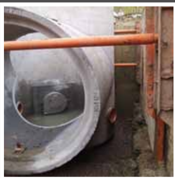
1600mm off 1600mm complete with pre-fitted Hydro-Brake® on headwall.
