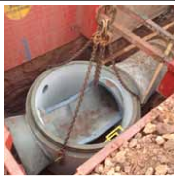
1800mm sealed chamber showing channel with slight bend
