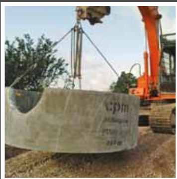
2550mm sectional installation, base chamber complete with half formed hole for 750mm pipe.
