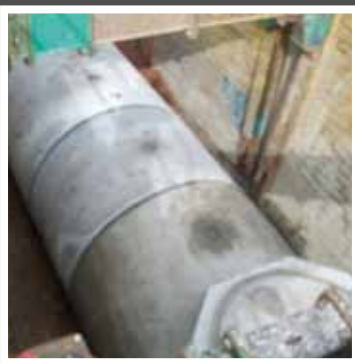
1500mm mid entry manhole
