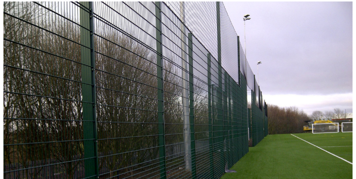
CODI "H" REBOUND INSTALLATION (ABOVE)
