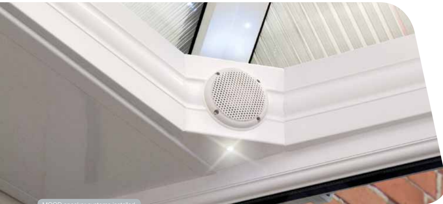
MOOD speaker systems installed
