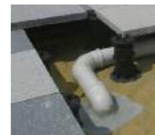
At roof level, DPH pedestals are used to support stone pavers to contain and protect the services for ventilation, water supply, lighting etc.
