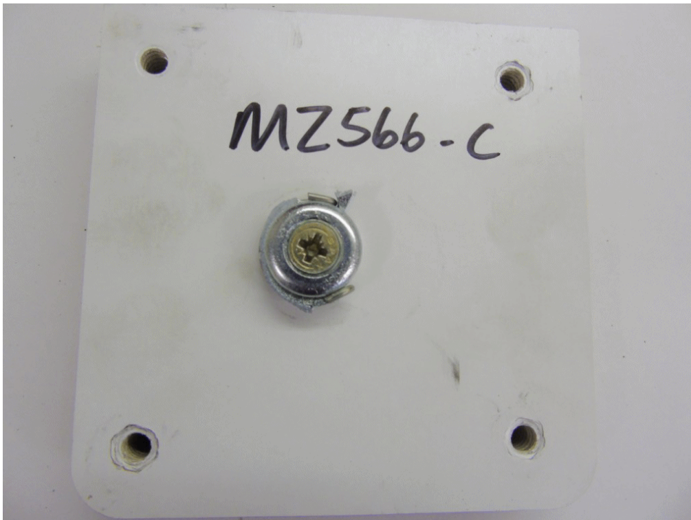
Photograph 6 A view showing the general condition of the button after a pull apart test on a type 1 - metal fixing.
