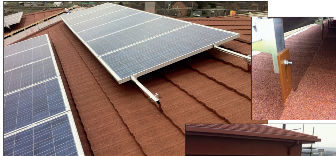
This project is a flat to pitch conversion, with Ultratile in Rustic Terracotta, and a Solar Photovoltaic system. All are supplied by Britmet Tileform Ltd.
