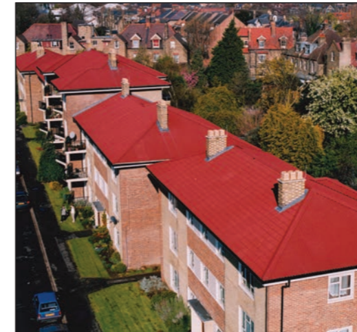
Boldroll ridge to eaves sheets can be fixed to a steel/timber sub-structure as in this flat to pitched roof conversion.
