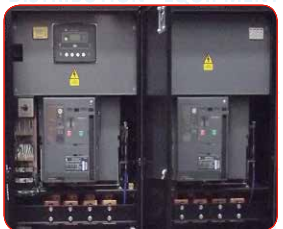
2000A AMF Panel Inset panels removed
