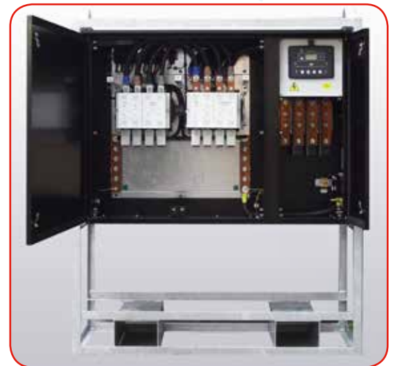
800A AMF Panel Inset panels and shrouds removed
