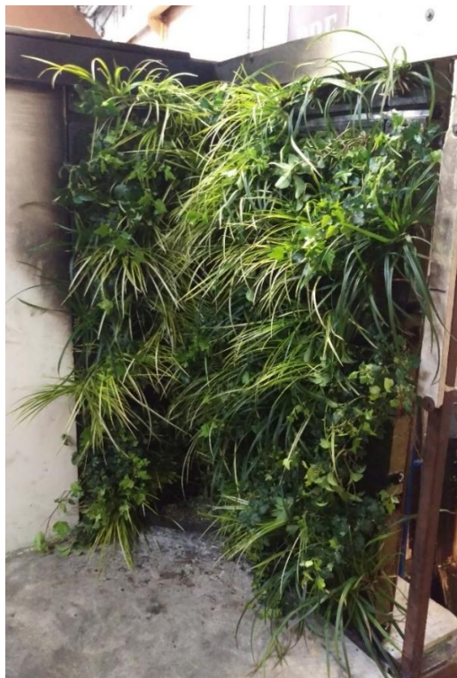
Photo 2 – Living Wall System before test 1 of BIO-FT-001 – Note the planted material cut back at flame impingement area.
