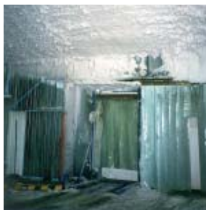
Icing-up leads to dangerous situations.
