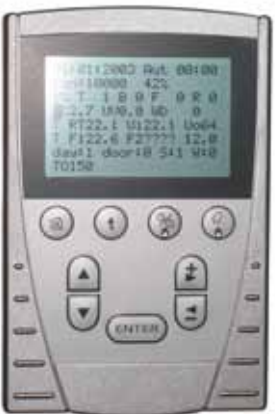
The PLC-service panel is part of the automatic control.
