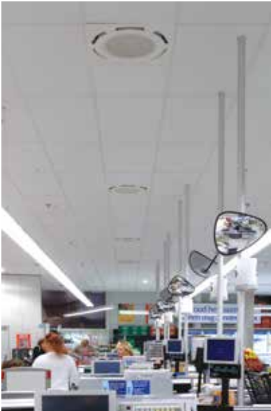
Cassette units (CC 60) installed above the tills at a supermarket.
