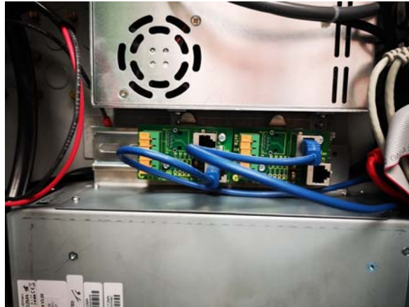
Figure 3.1 — Internal view of the Local Control Panel
