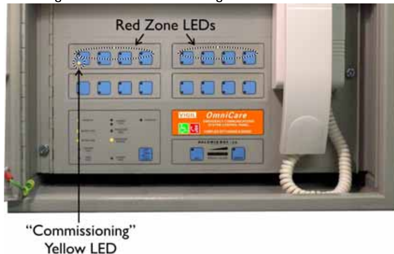
Figure 4.10 — Commissioning Process LEDs
