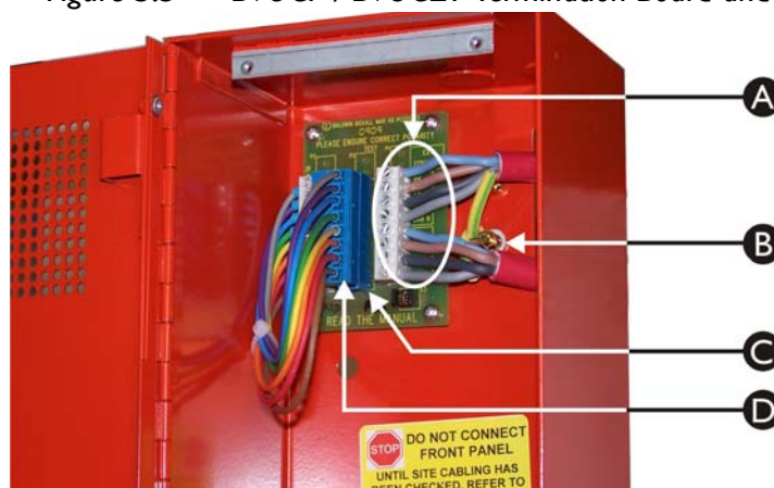
Figure 3.5 — BVOCF / BVOCET Termination Board and Site Wiring
