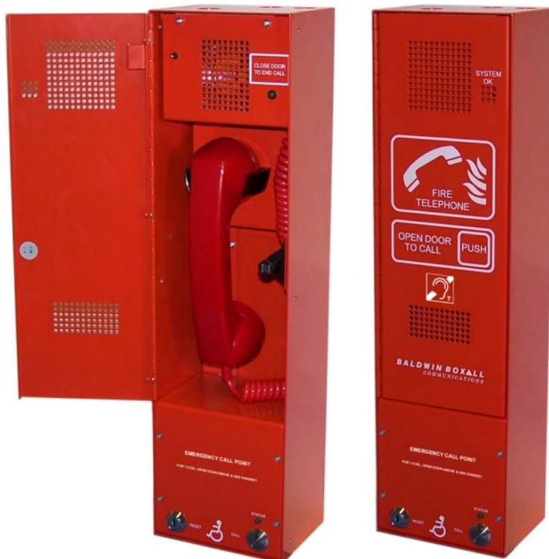
Figure I.5 — Typical Combined Disabled Refuge / Fire Telephone
