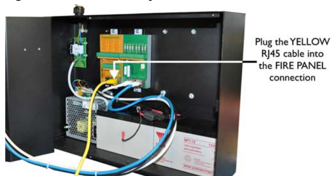
Figure 2.13 — Yellow RJ45 Cable connected to C2CFPE
