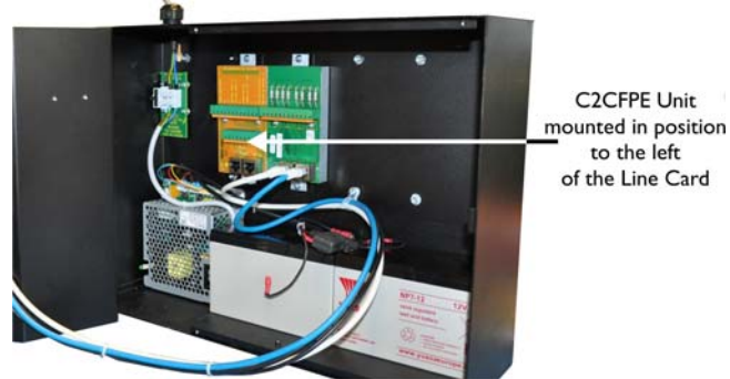
Figure 2.12 — Internal View - C2CFPE unit mounted in position
