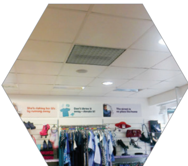
SCHG-30 installed in a charity shop in Calverton, Notts
