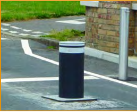
Automatic bollard at Marshall Aerospace
