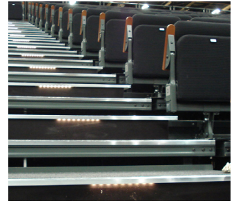
Aisle Lights - Low voltage, low glare, LED lighting with optional one hour battery back-up and dimming function.
